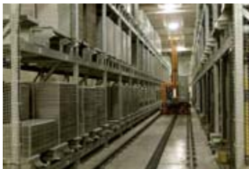
An automatic storage/retrieval unit handles the bakery's inventory of 26,000 bread pans. Reduced labor and extended serviceability of the pans are among the system's advantages.
